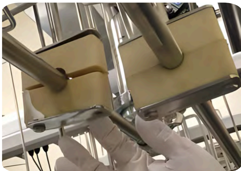
Image Details: Loose or missing supports lead to slope issues, raising contamination risk
